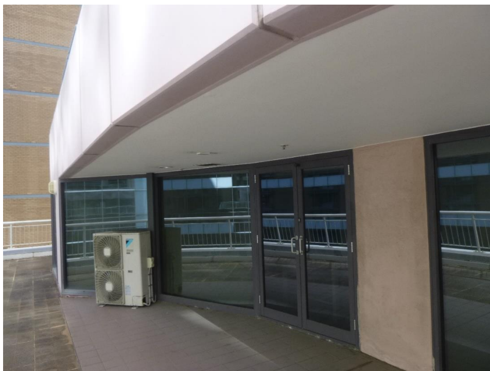
Plate 8 – Level 11, exterior western terrace, ceiling – fibre cement sheeting. NAD Date: 09/03/2018
