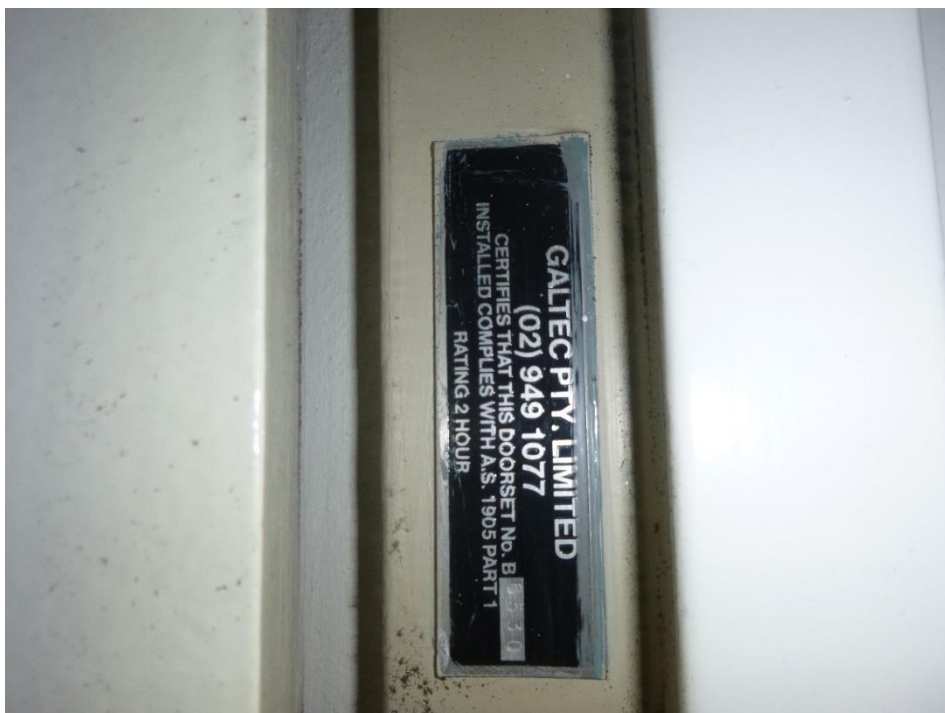
Plate 2 – Levels 1 – 11, fire escape stairwells, fire doors – suspected asbestos-containing fire door core. No definitive markings present such as manufacturing or installation data found on newer fire doors. Date: 09/03/2018
