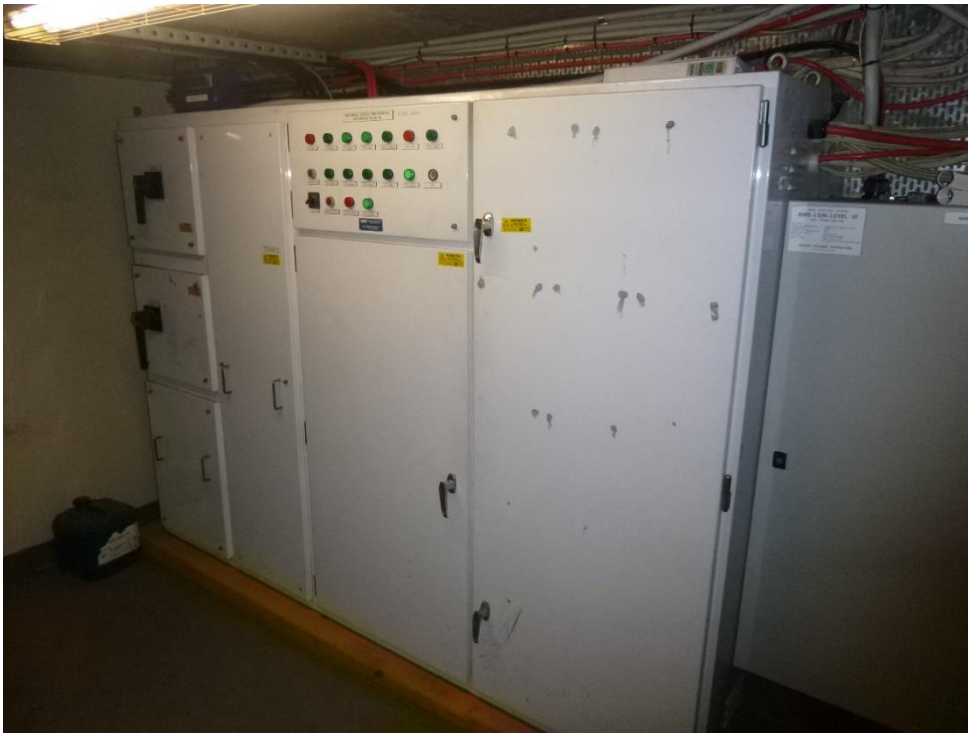
Plate 3 – Level 12, plant room, central area, electrical board “Mechanical Services Non-Essential Switchboard No. SB-12A” wide angle view of the whole panel enclosure.
