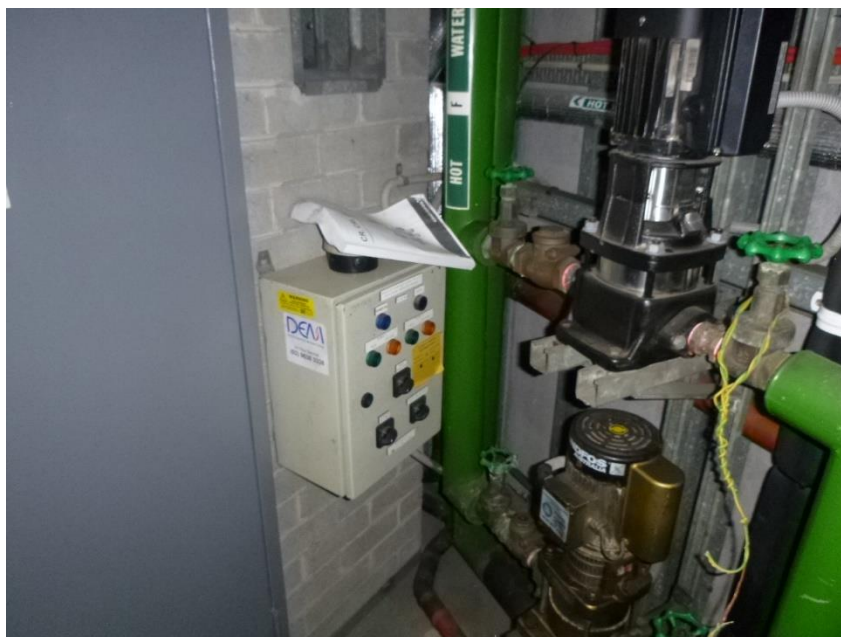
Plate 5 – Level 12, Plant room – north western area, adjacent double doors to Hydrant Diesel Pump Not sampled due to Live Electrical Hazard.
