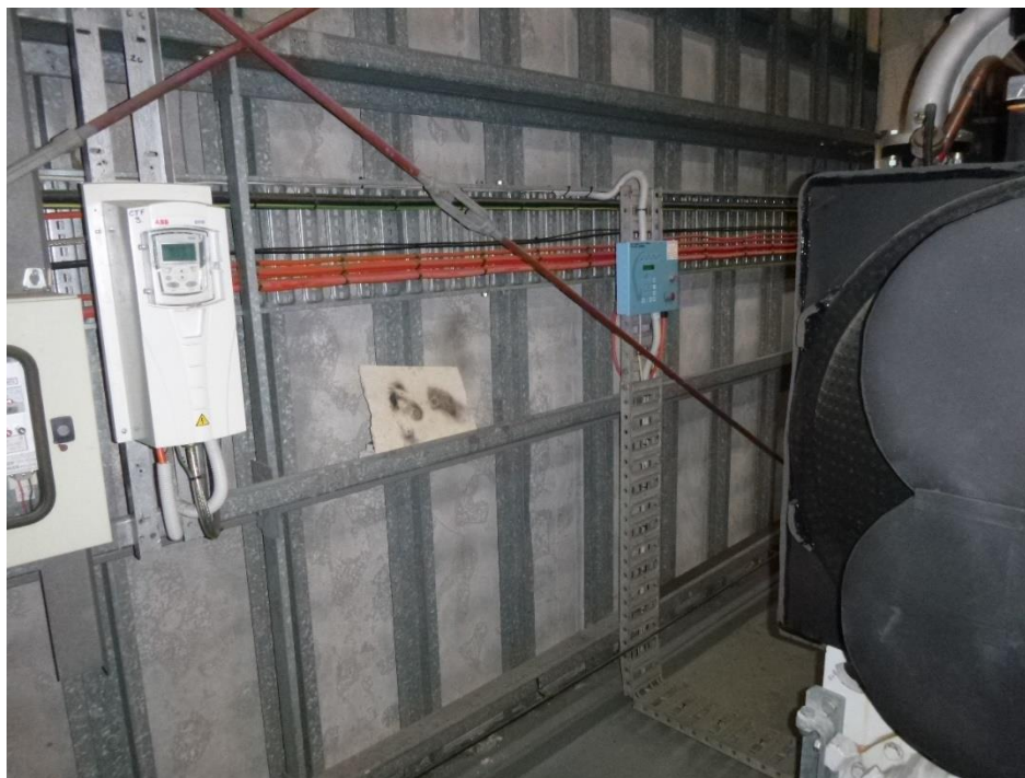
Plate 7 – Level 12, Plant Room, southern wall ledge adjacent to Chiller No.1. Fibre cement debris. No Asbestos Detected ('NAD') Date: 09/03/2018
