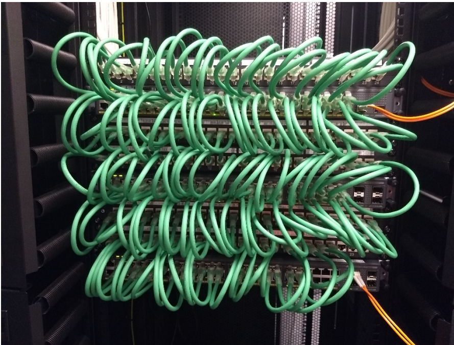
Figure 6.1.8.1 – Example Patching of rack
